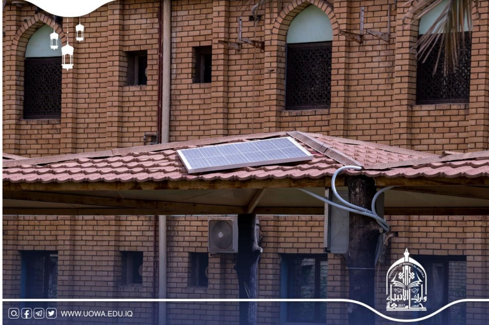
Solar panels over shades for charging e-devices (General use)
